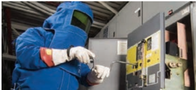
Figure 3 - check of covers, doors and all bolts
